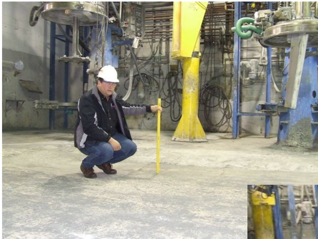
Above – low area causing Unsafe operating condition
